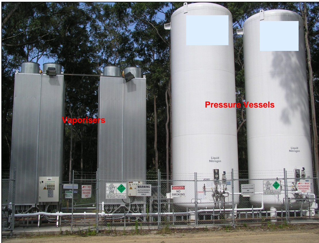
Figure 28: Ambient Air Vapouriser
